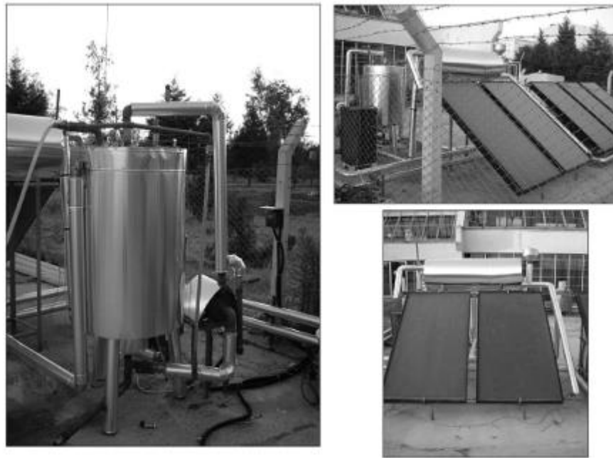
Figure 12 Solar heated biogas system (Koçar and Eryaşar, 2007).
